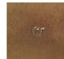
f) partially removed scab
