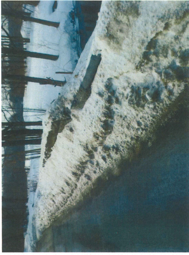
Photo #: TYPICAL PARAPET SNOW COVERED. WEST END SHOWN
